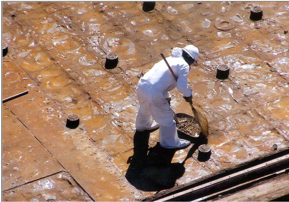
Photo courtesy of Laura S. Johnson Worker sweeping debris during flight deck removal onboard the ex-USS Oriskany.
